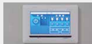
On-site Lighting & HVAC Control
