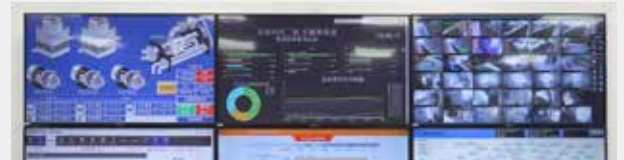
Central Control Room Remote Monitoring
